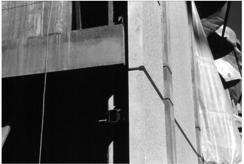
Figure 5.2.6. Pre-cast panels assembled on a concrete frame, showing joint detail and tolerance gap between panels and floor slab.
