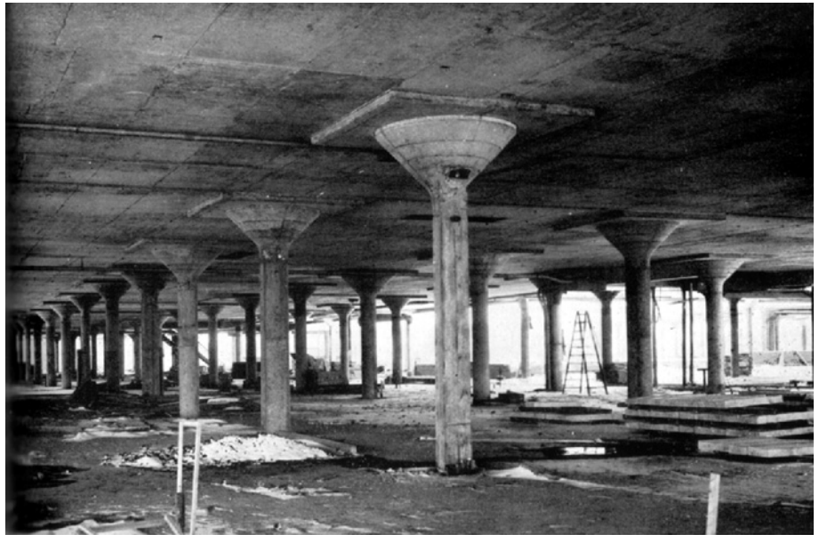
Figure 4.6.2. One of the limiting factors in slab design is the high shear stress that can develop between a flat plate and a supporting column. A typical solution is to spread the column out at the intersection and/or to add a flat drop panel. Both of these have the effect of spreading the shear across a wider area – the cylinder that is formed by the circumference of the column capital and the depth of the slab. From Leonard Michaels. Request sent to Reinhold.
