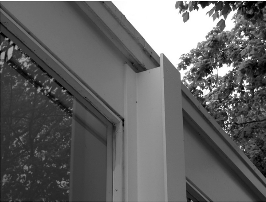
Figures 5.5.7 and 5.5.8 Mies van der Rohe's Farnsworth House in Plano, IL, is a minimalist pair of planes with living spaces perched tenuously between. To emphasize the crisp, tight spatial concept, connections between steel columns and beams were welded and ground, so that no bolts or connections are visible. Steel window frames were set just inside the structural frame, offering a very subtle – almost unnoticeable – hierarchy.
