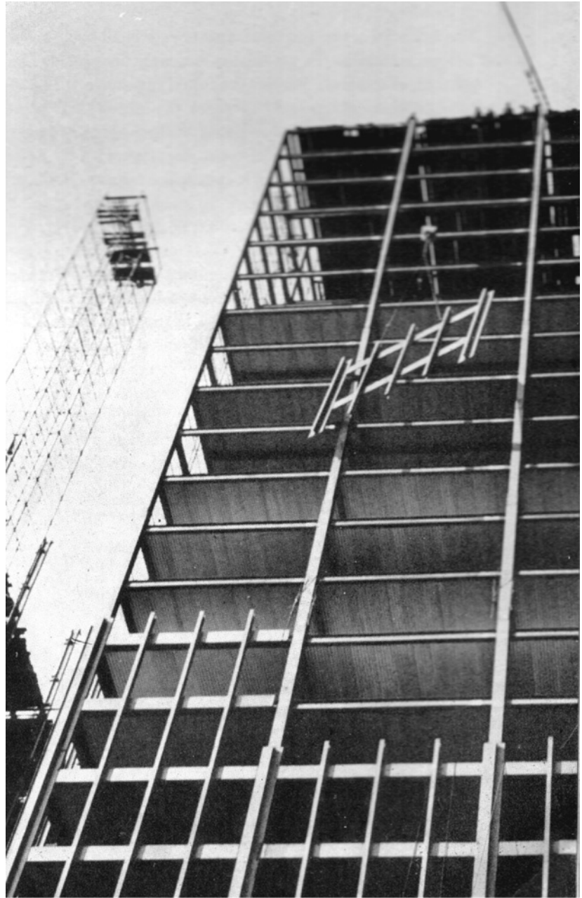
Figure 5.2.2. A clear demonstration of the curtain wall's configuration and assembly; a panel is lifted into place on Mies van der Rohe's 1949 Lake Shore Drive Apartments, to be filled later by glass panes.
