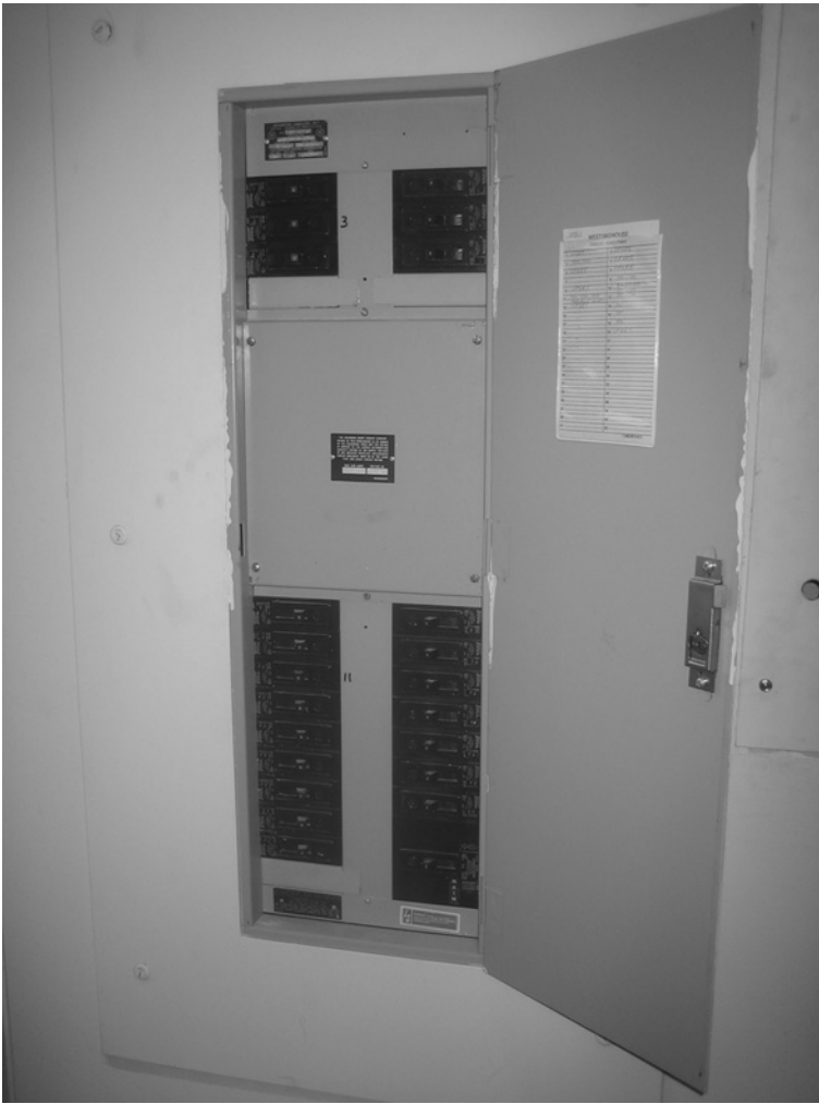
Figure 6.6.5. At typical panelboard, which serves as both a distribution panel and a central point for disconnecting individual circuits.
