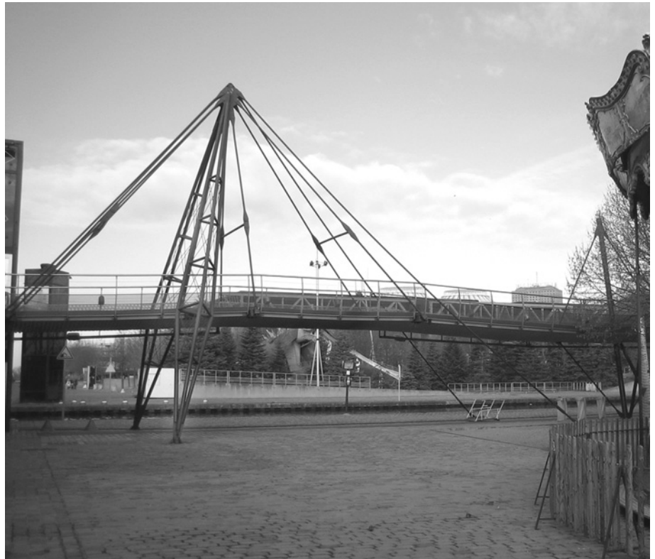
Figure 4.5.8. A structurally expressive skylon, wider at the middle to counteract buckling forces at La Villette, Paris. Bernard Tschumi, Architect; Peter Rice, Engineer.
