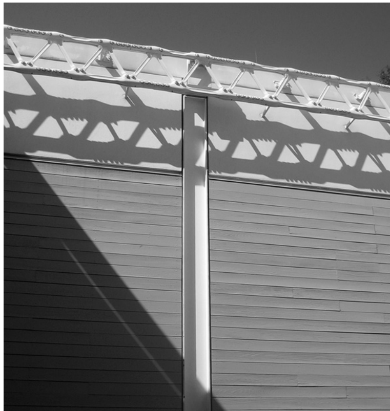
Figure 5.5.10. Renzo Piano's Menil Museum in Houston, TX, fit simple wood siding into a steel frame, allowing it to relate to the clapboard houses in its neighborhood. The boards are aligned with the front of the column's flanges, so that the beam's indentation creates a reveal, or break, in the wall. Elements of the roof form overhead show the building's internal rhythm.
