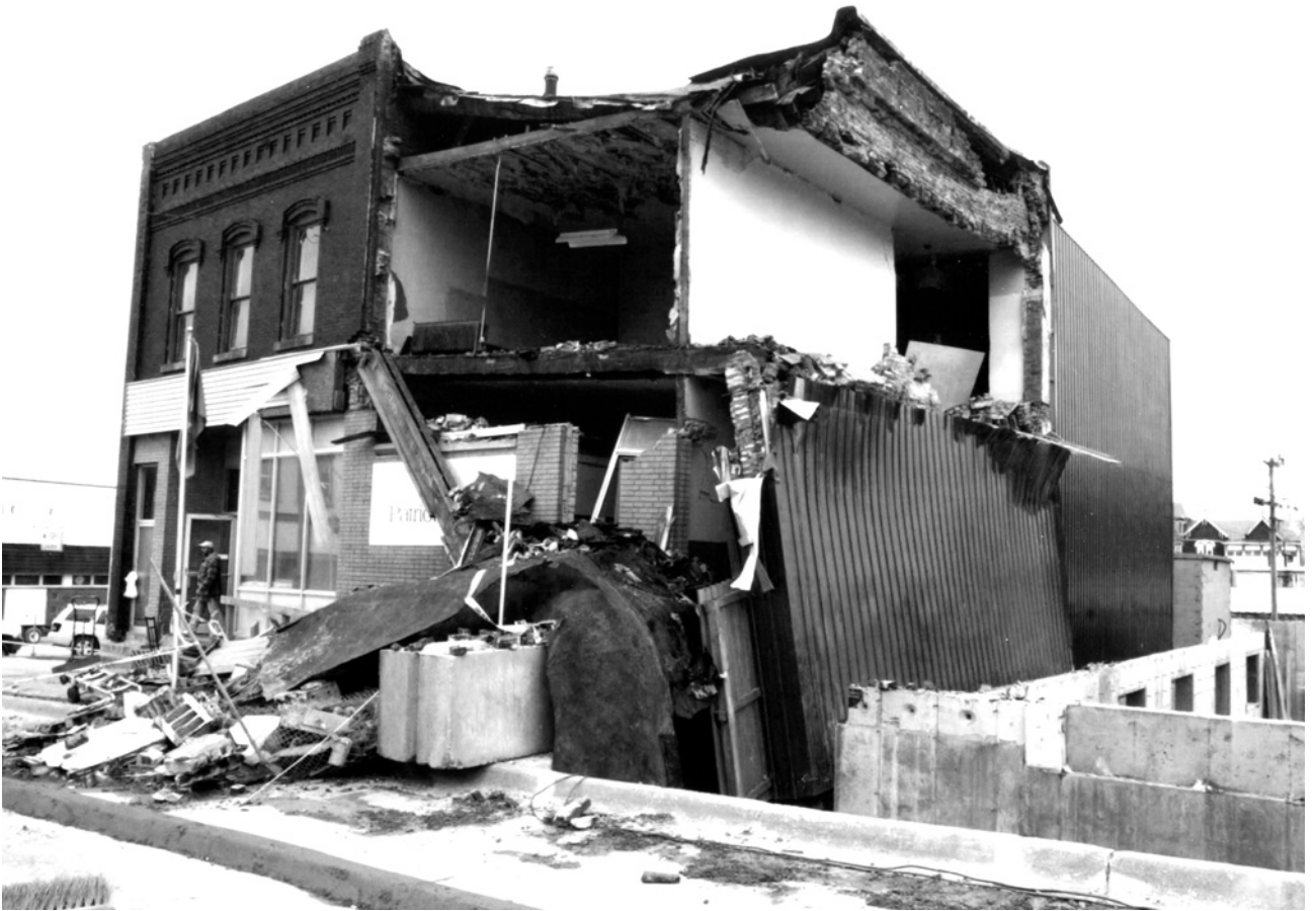
Figure 4.7.9. What happens when foundations go bad. In this case, neighboring construction allowed the soil that had supported this bank building to slide. With nothing to bear upon, the footings collapsed, bringing down most of the building with it. (Des Moines Register).
