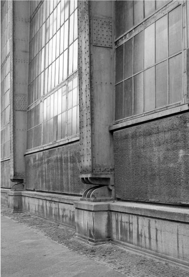
Figure 5.5.11. Detail can be structurally expressive. Here, Peter Behrens AEG Turbinfabrik in Berlin (1909) used steel ‘knuckles’ to allow the frame above to move without disrupting the foundations. Behrens obviously recognized the chance to put this structural principle on display, attaching the knuckle to a bench-like base and slipping the factory windows behind the steel frame.
